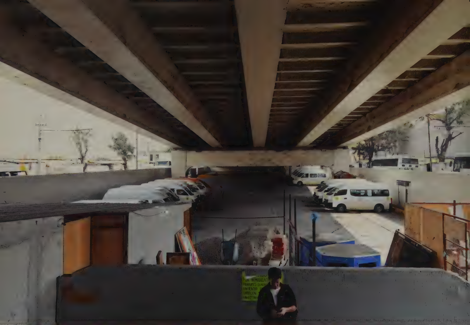
9:07 Beneath this underpass, unseen, it is time to descend further below. The sign for the metro station is hardly visible. The handrail along the stairs is missing and the marble floor tiles, the ones that become dangerously slippery in the rain, are chipped. Once again, I almost didn't notice the plywood construction shacks in the background. They've been there for a while.
