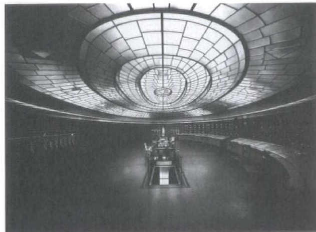
Tivadar Kozelka, Helenföld Power Station (arch. Virgil Bierbauer), Budapest, 1927–33. Control room, long axis.
