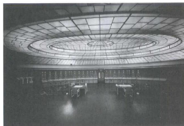
Tivadar Kozelka, Helenföld Power Station (arch. Virgil Bierbauer), Budapest, 1927–33. Control room, short axis.
