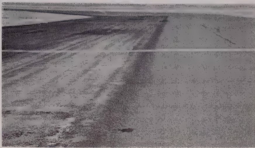
ASPHALT-CONCRETE taxiway shoulder at Edwards Air Force Base with 0.15 gsy. of a 4:1 dilution just applied at left. Note excessively dry and pitted surface and large shrinkage cracks in background. Pavement, about 6 yr. old, receiving treatment just barely in time as surface beginning to ravel and becoming quite rough. Over 400,000 sq. yd. of such pavement treated to date with 50,000 gal. of Reclamite concentrate. Note pavement markings still visible in treated area.
