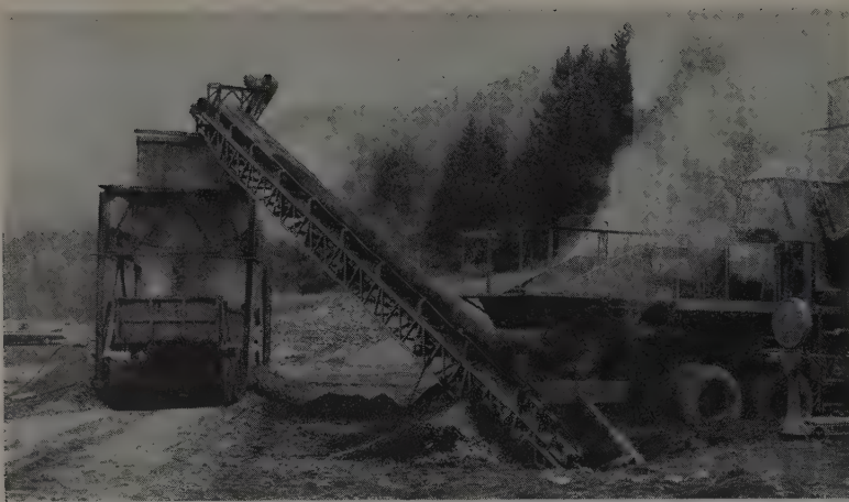
A FEATURE of the plant was the 30-ton surge bin for the hot mix, which reduced time for truck loading, cutting at least one unit out of the hauling fleet. It also solved another loading problem since drive-through loading under the pugmill would have been below ground-water level.
