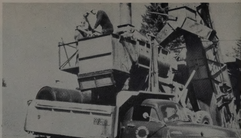
FROM THE ELEVATOR the aggregate drops into the pug mill for a mixing interval estimated at 14 sec. Emulsified asphalt is 4% of the weight of the aggregate. Output of the plant was 120 tons per hour as compared to its rated capacity of 60 tons of plant mix.
