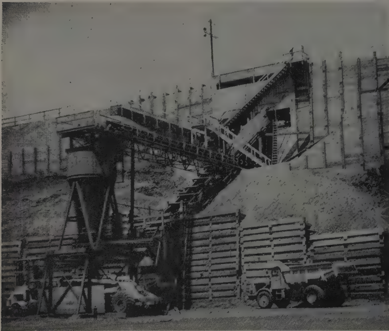
CLASSIFYING SYSTEM feeds minus 3-in. material to horizontal conveyor which brings it to silo for loading into bottom-dumps. Plus 3-in. slides down chute into rear-dumps.
