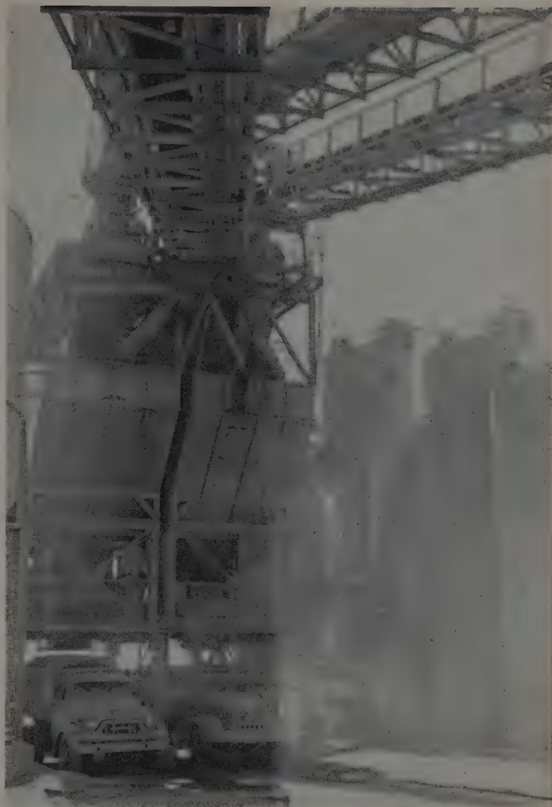
DOUBLE BATCH PLANT , which can produce 600 cu. yd. per hr., loads two trucks at once. The plants are Conveyco, one with a 325 yd. per hr. capacity, the other with 275. The plants are completely separate, each fed by a 400-ft. long conveyor (see cover).
