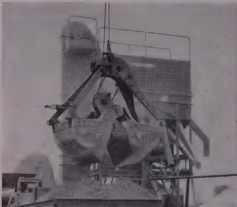
ERIE rehandler shown charging hopper of rotary drum dryer unit of the Gregg County Barber-Greene Asphalt plant.
