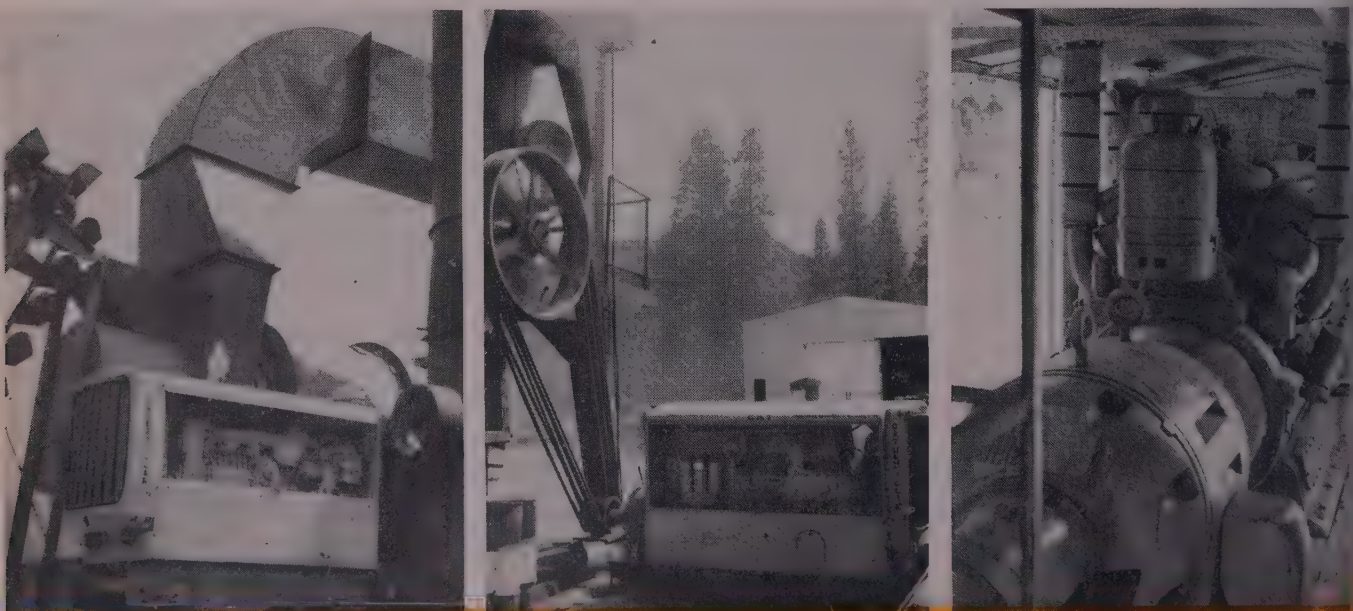
Three Cat Diesels power the Standard Steel hot mix plant: A D318, left; D342, center; and a D364 Electric Set, right.
