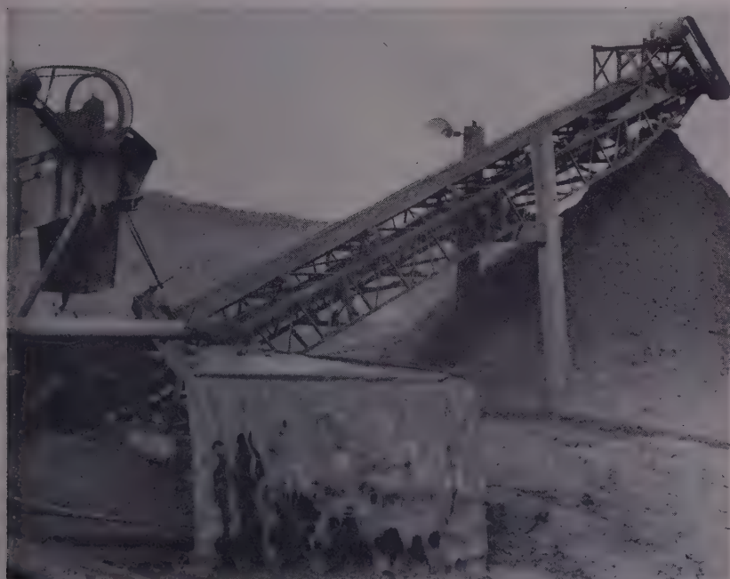
RECLAIMING washwater was a feature of the plant operations. Dirty water shown emerging from the Eagle sand dehydrator flows to a stilling basin from which it was reused. The problem of adequate water for washing gravel is a typical Western problem.
