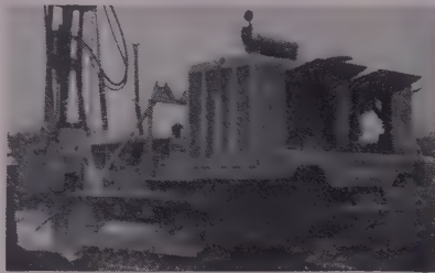
Calumet-Sag Channel —G-D rotary compressor furnished air for tractor-mounted drill.
