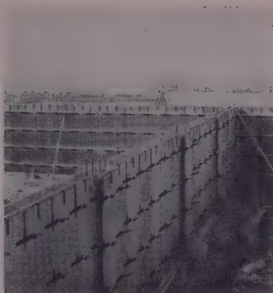
LARGE THEATRE in Alaska—Note minimum alignment and bracing.
