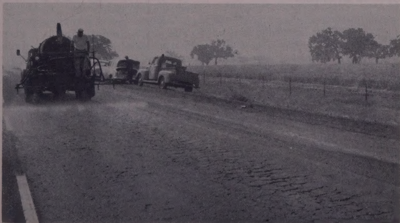
LIMITATIONS OF SLURRY SEAL must be understood as well as its capabilities. In the case shown the blocks formed by alligator cracking were moving under traffic. Slurry seal did not correct.
