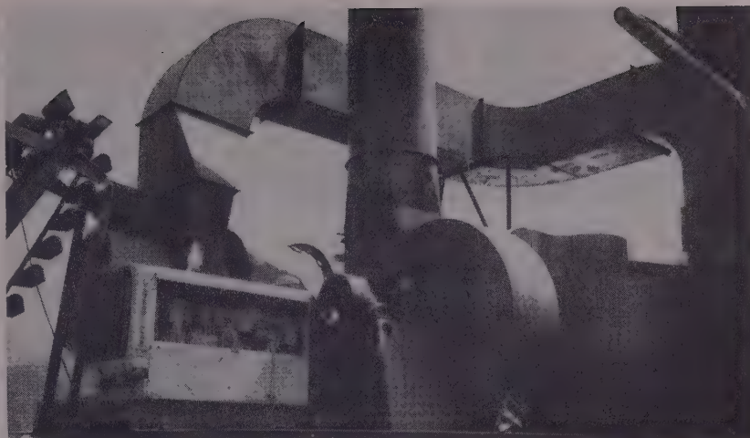
CRITICAL CHECK POINTS in preventive maintenance for asphalt plants are the blower and cyclone. Uneven or unusual wear on the blades causes vibrations to be transmitted back to the motor.
