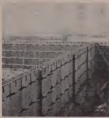
LARGE THEATRE in Alaska—Note minimum alignment and bracing.
