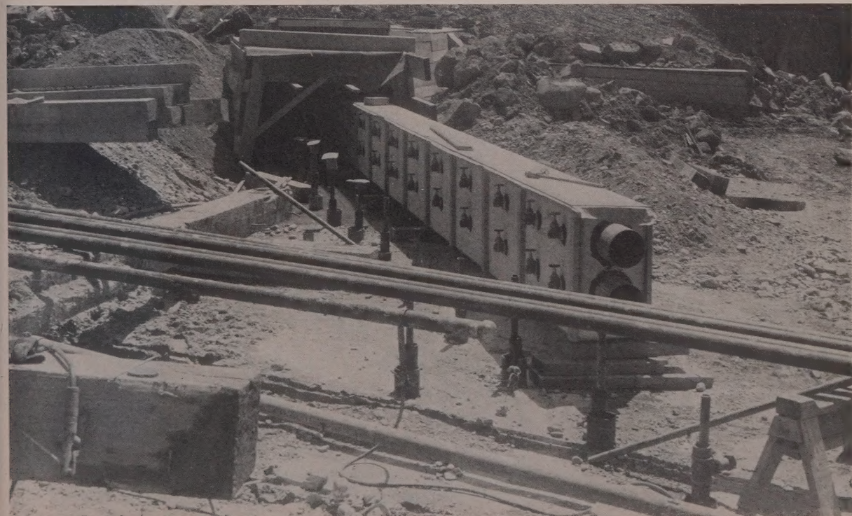
ENCLOSED in the insulated box are a 10-in. brine supply line and the return header. The freeze points are shown projecting out of the 6-in.
