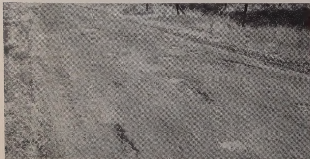
Fig. 1—Condition of the road before the start of improvement program. Note the lack of elevation, with irrigated fields on both sides. More than maintenance was required and cost was a governing factor.
