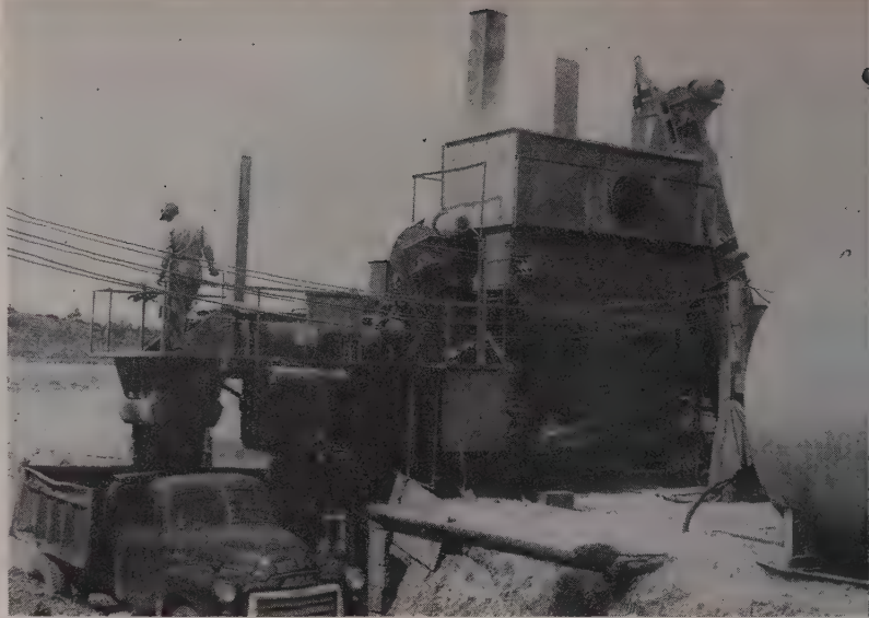
ONE OF TWO control stations for operating the entire plant. The other is near the burners at the drier. Dumping from the Continuflo surge hopper eliminates segregation of the mix. Bitumen is an 85-100 penetration asphalt.
