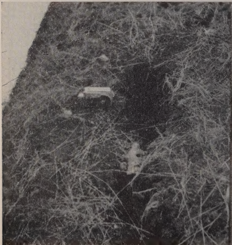
CAUSE —Soils that have this much volume with wetting-and-drying (note camera showing size) will produce a serious effect on the sloping concrete lining of a canal.
