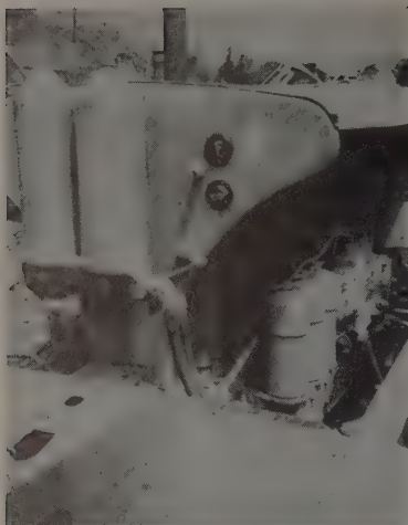
SUPPLEMENTING the regular filter installation, additional units (left) provide a factor of safety under tough conditions.
