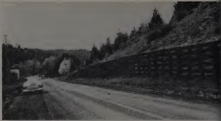
CRIBWORK of pressure creosoted timber is effective in holding slides without preventing drainage. This example is on the McKenzie Pass Highway, Oregon Route 28.
