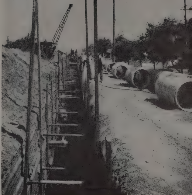
ADEQUATE TRENCH shoring costs money but the savings always exceed the costs. Only one out of thirty accidents results in injury but they all are full of expenses, most of them hidden.
