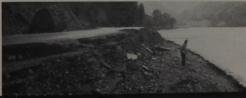
BELOW —Sacked concrete rip-rap along the Eel River at Greenlaw Bluffs kept this embankment from washing out entirely. When this section was built years ago the rip-rap was placed 5 ft. above the highest recorded stream level. During the Christmas flood the water was over the roadway at the upper left.
