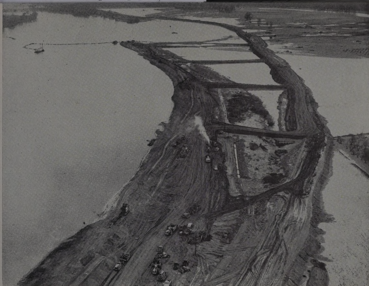
THE mile-long new levee bowed out around the break to avoid the deep channel the water scoured when pouring through the gap. This
