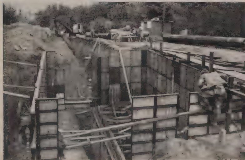
TACOMA RESERVOIR WILL HOLD 50,000,000 GAL.
