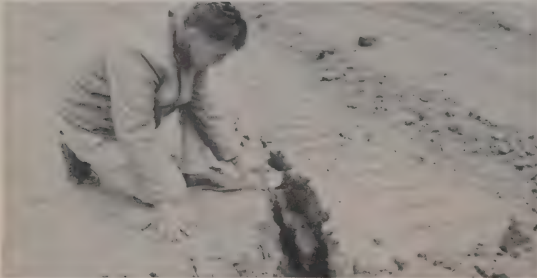
SHEAR CRACKING was curse of comparative rolling program. This happened along edge of test embankment, indicating vertical boundary and possible lateral movement.
