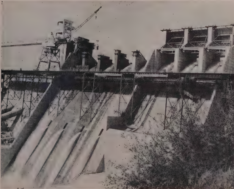
PRODUCING POWER BEFORE COMPLETION
