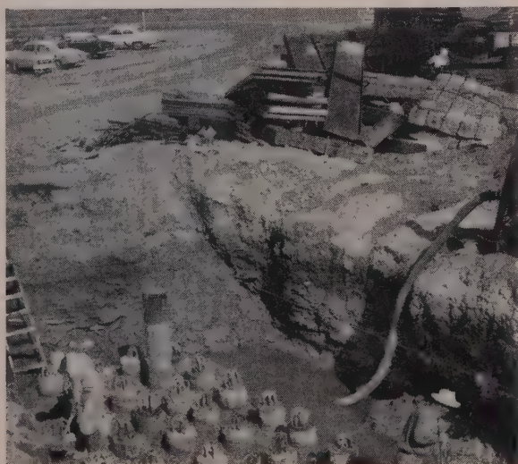
RAYMOND STEEL-SHELL pile cluster for pier foundation lies in hot, corrosive sulfur water. Water table was only 4 ft. down.
