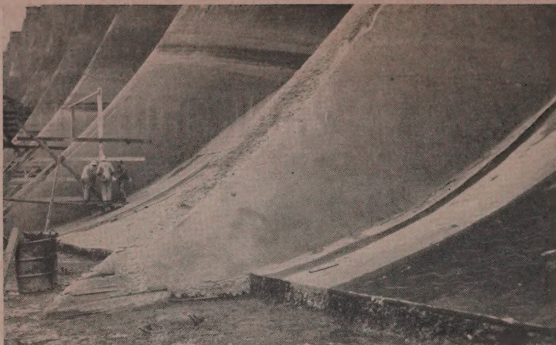
EROSION AND CAVITATION damage had attacked pier noses, baffle deck and baffles. Deck was cut back as shown below ogee to insure good bond for new concrete.
