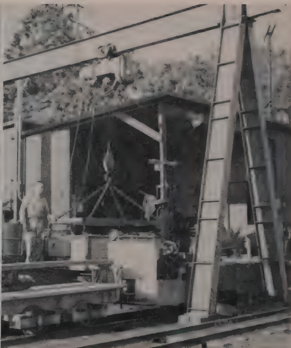
MECHANIC GEORGE EASTON runs an efficient maintenance shop at the south portal. Battery changes on the Goodman locomotives are made every 6 hr. running time with use of gantry hoist shown here.
