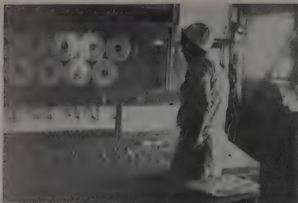
NERVE CENTER for all operations is the control room of the Johnson automatic batch plant. Merely flicking a dial sets new batch weights for a different mix design. Invaluable is a moisture compensator.
