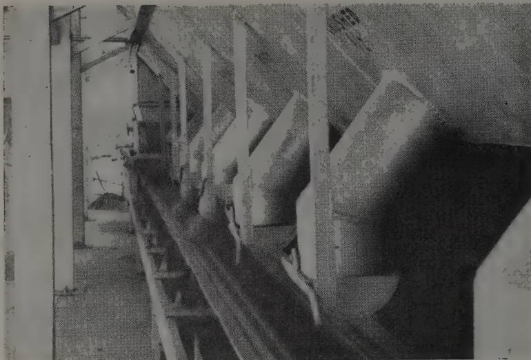
ADJUSTABLE COARSE AGGREGATE feeders are of the gravity type such as shown here. They have a positive locking pin. Belt feeders or vibrator feeders are usually used for fine aggregate. Aggregate sizes are noted on the bins.
