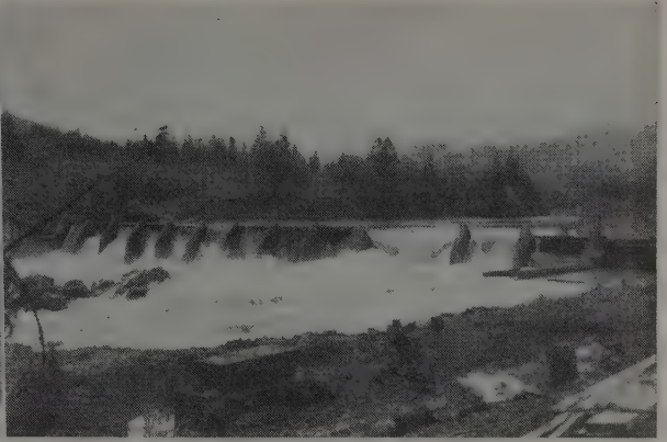
MAY 27, 1953 —View taken from the south bank the day after upstream cofferdam failure. River flow of 20,000 cfs. made a shambles of the sheet steel piling. Flow in picture is 12,800 cfs.
