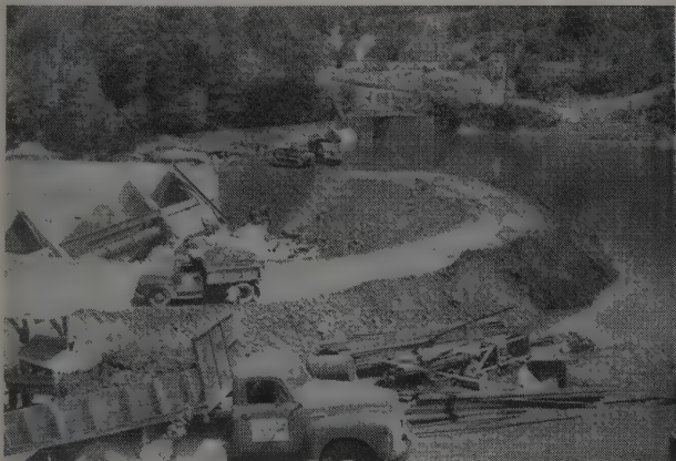
JUNE 30, 1953 —Cofferdam No. 2 failed on June 24, washing out 125 ft. of the midstream section. It is being rebuilt here using old concrete piers, quarried granite, and an upstream clay blanket.
