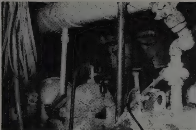
PUMP STATION is no place for camera panorama! Main units are Fairbanks Morse and Ingersoll-Rand centrifugals, jammed in to boost more than 6,000 gpm. from sump to portal 2 mi. away.
