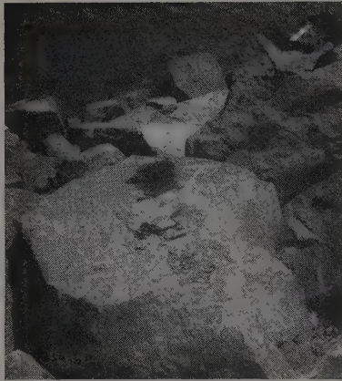
BEFORE blasting, wide gaps between rocks permitted waves to wash out gravel blanket underneath.
