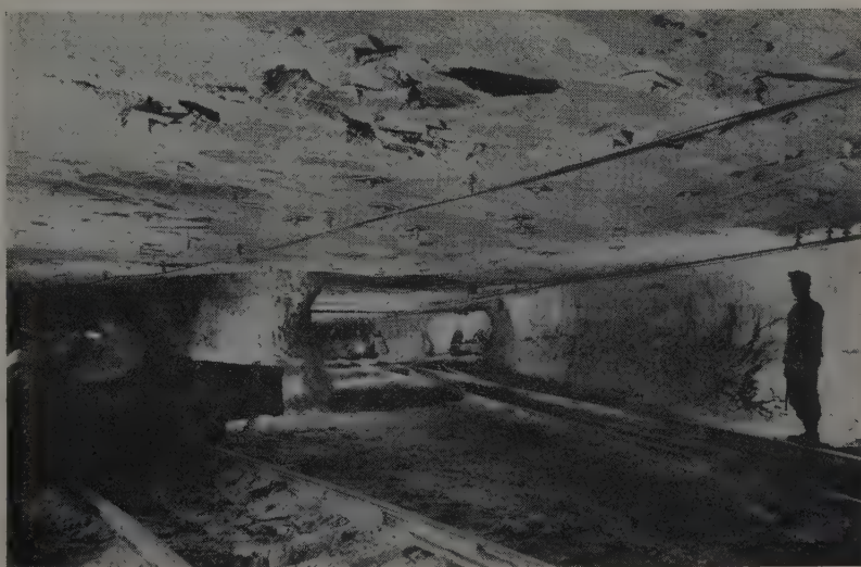
LAMINATED BEAM supporting extremely wide roof spans is formed when rock strata can be tied together by bolting. This haulage-way installation represents a common bolt application in coal mines.
