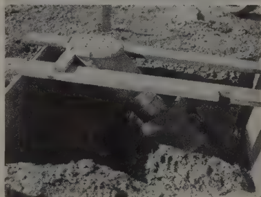
INTERIOR of the main garage (top) shows the overhead door at one end. Mike Sienert, Power District civil engineer (center), shows how gas fumes will be eliminated for more safety and convenience. A closeup (bottom) of the exhaust gas vent, taken before the concrete slab was poured.
