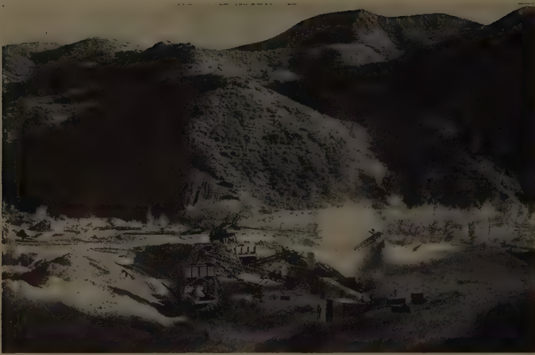
THIS 46VE plant turned out more than half a million tons of base course and hot mix aggregates for Winston Brothers to use on 40 mi. of the world's toughest mountain construction, knocking out the curves on California's famous Ridge Route.
