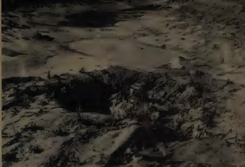
PIPING through earth lining resulted from drying shrinkage and frost cracks after canal had been emptied for construction work.
