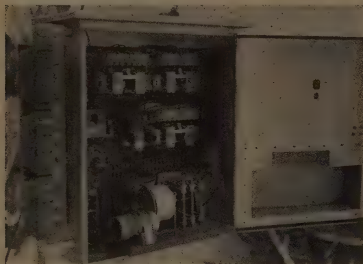
THE RECEIVING UNIT, located in the electrical cabinet on the lower wing wall of the headgate structure, shown here below the control panel.
