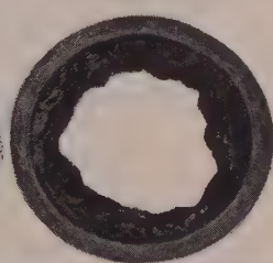
Typical pipe line before Pipe Linings treatment
