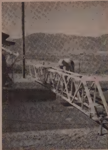
SPANNING the test track between precisely leveled support pins, the profilometer (above) enables reference of transverse profile records to the project datum.
