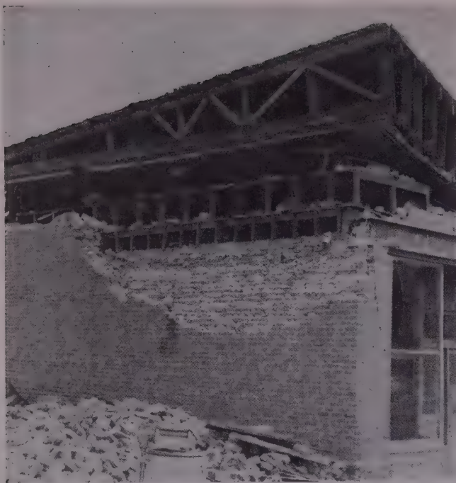
TYPICAL FAILURE of poor workmanship and faulty materials is shown in this bearing brick wall in Tehachapi. Weak mortar and unfilled head joints were common. This second story apparently housed a meeting hall; roof is now supported by grand piano and auditorium chairs.
