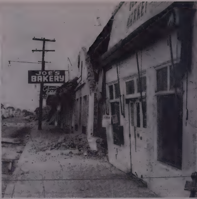
THE OTHER SIDE of the main street in Arvin looks just like this, if not a little worse. Though badly bulged, building front in foreground still stands. Poured bond beam above door may have helped, but not enough. Estimate indicates 50% of city's downtown buildings will have to be condemned.
