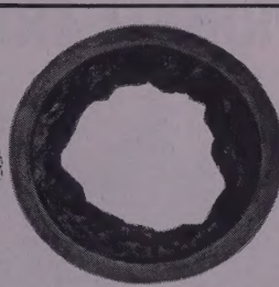
Typical pipe line before Pipe Linings treatment
