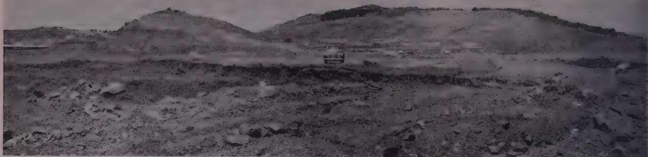
ABOVE: Sudden settlement at Sta. 16+00 occurred after nose of fill had advanced well ahead. Borrow area in left background.
