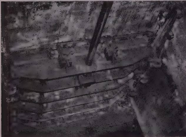
LEFT: Looking down at one of the sluice gates. It is 6 ft. wide, 5 ft. high, with a rising stem. Weight: 2,900 lb.
