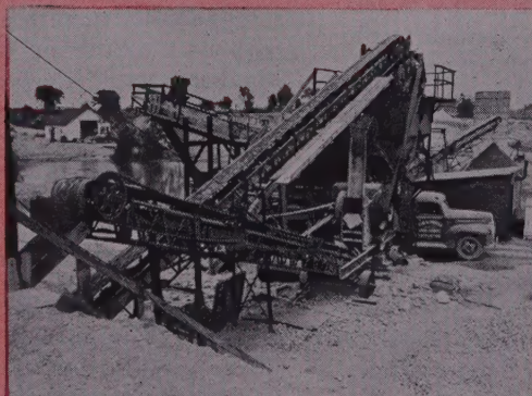
Return conveyor provides closed-circuit operation
