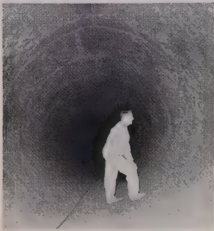
CONDITION of Placerita Siphon after cleaning. Propeller-type cleaning machine used short lengths of chain to dislodge loose material.
