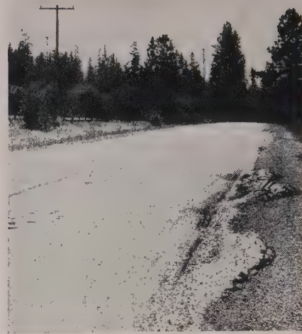
RUTTING and shoving a bituminous surface may result from repeated heavy axle loads. In this case, a majority of loads traveled in the right-hand lane, and lack of distortion in the other lane was evidence of the cause of damage.
