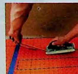
Schluter-Systems Bathroom Installation & Floor Heat schluter.com
