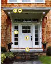
Sheltering a wood door from the weather helps preserve its looks and increases its life span.
