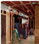
Wrapping foil-faced fiberglass around metal ductwork helps it resist banging noises when the furnace is operating.
