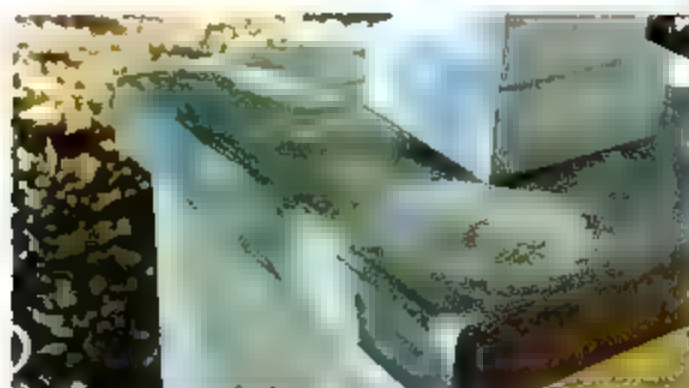
The constant wetness of a potted plant probably created the circular blemish on this concrete porch pier. TOH general contractor Tom Silva recommends a cover-up.
