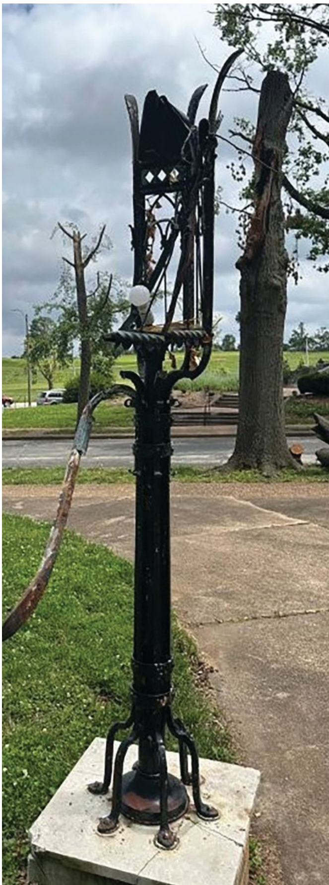
EXTERIOR FIXTURE DAMAGED DURING 2025 TORNADO
