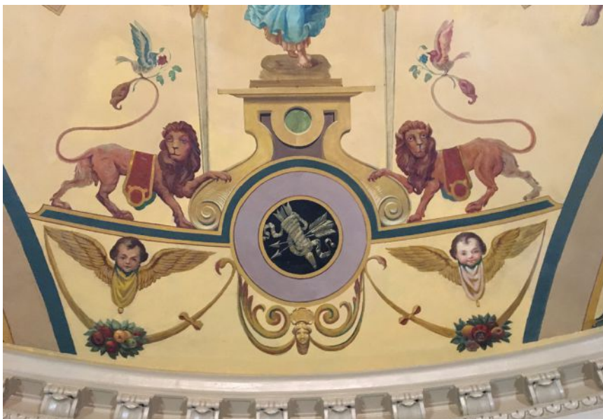
ABOVE Paint loss was most severe on plaster substrate areas, where water infiltration had caused delamination. Conservation included re-attachment with adhesives and in-fill painting with modern, reversable materials.
