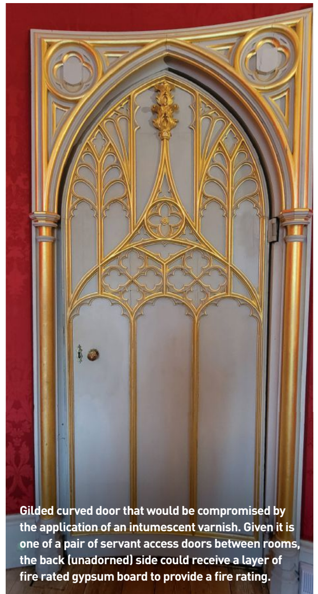
A historic door that could not be made to meet ADA spatial requirements for width or pull side clearance. By planning use of the building differently, access to the space beyond was made through another path not requiring modifications to the historic fabric.
