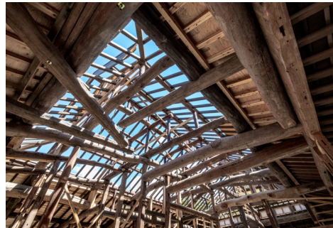
The original roof beams were used whenever feasible in the reconstructed framework of the house.
