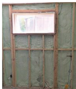
Post flood, drywall is removed and Demilec insulation is intact.
