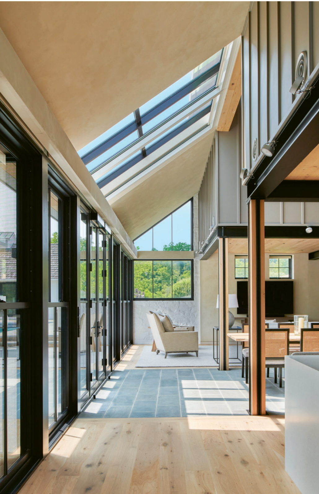
New steel framing supports a cutaway second floor, while a south-facing glass wall and skylights flood the living spaces with light. Beyond the living room are a new pool and perpendicular screened porch—the former manure shed.
